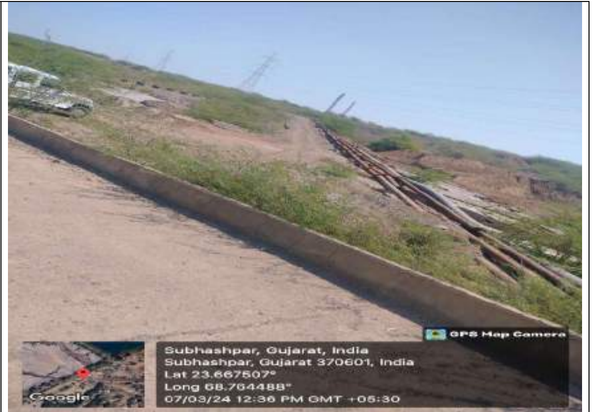
Fly ash slurry lines from TPP to Dyke-D
