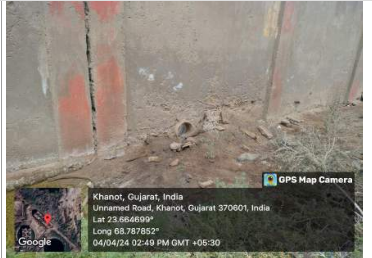
No flow outside units premises near cooling tower
